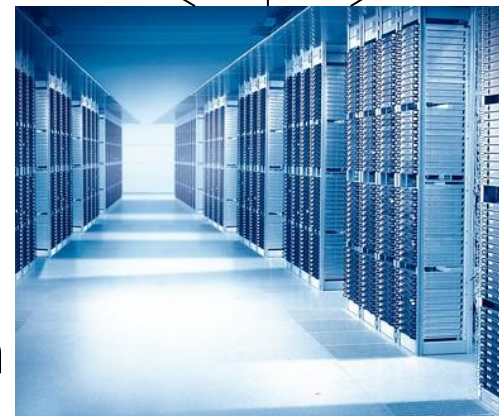
Strato Data Centre, cloud ^
